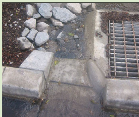
Figure C-15 Curb cut right next to the overflow.
