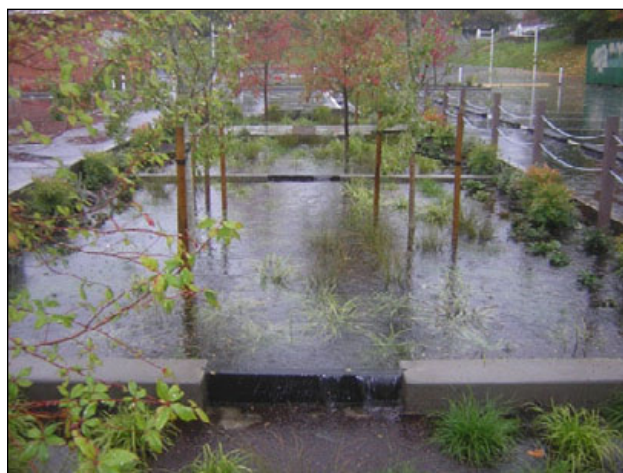
Figure C-26. Concrete check dam with an adjustable weir.
