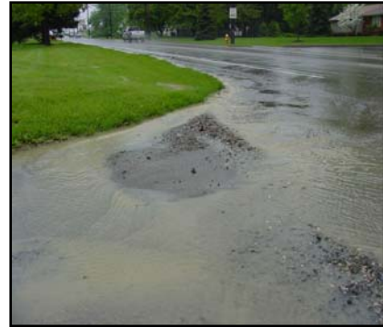
Excess impervious cover creates a landscape that cannot absorb or infiltrate rainfall.
